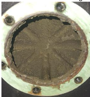
Before Chemical Cleaning
