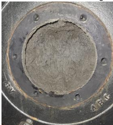
Before Chemical Cleaning
